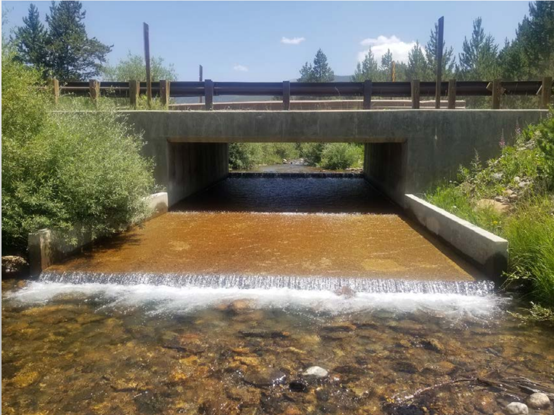
Ineffective Current Velocity Barrier
