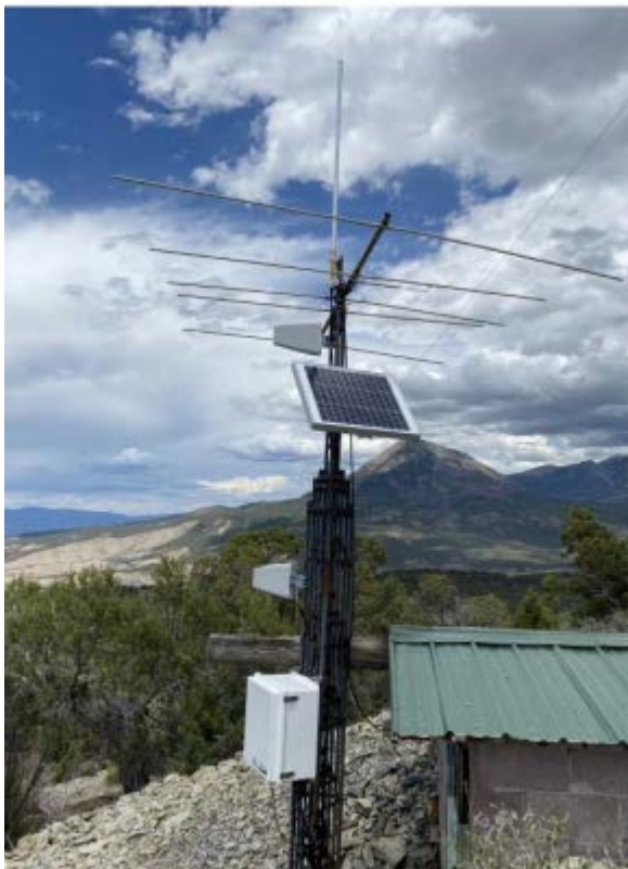
Figure 8 - Young's Peak Communication Station, Crawford, Colorado
